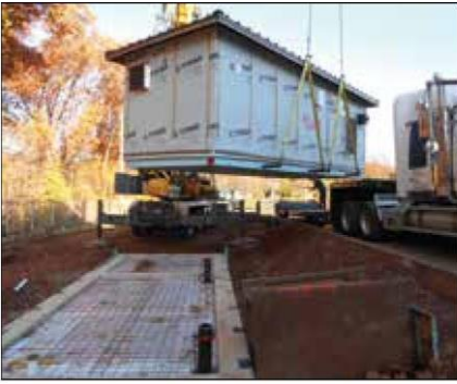
The new East Side Pump Station is set into place in Southington
