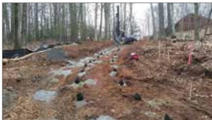
Preparations for blasting of the ledge along the proposed water main route
