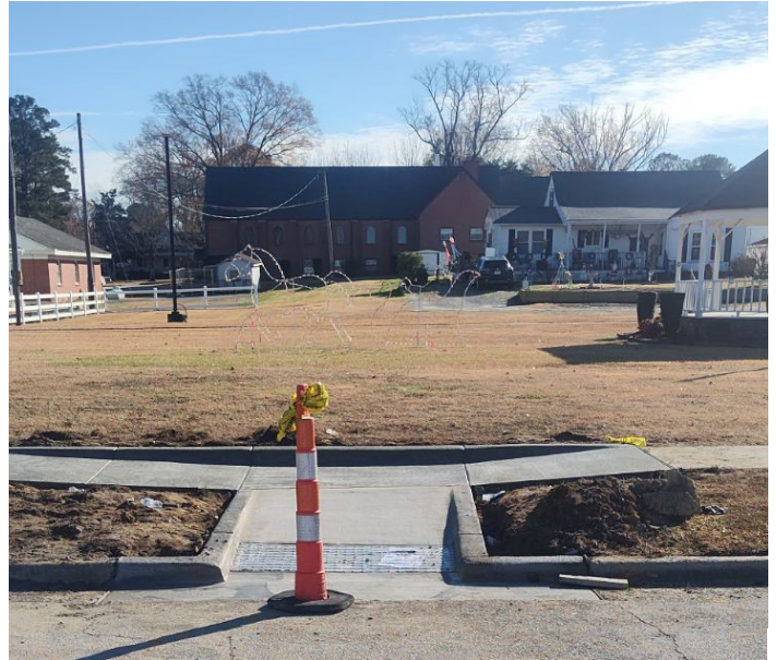
The image above shows a new curb ramp installed on the Town Commons to provide better access to strollers and wheelchairs.
