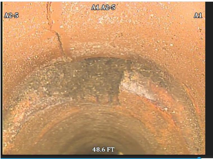
Picture of A1-A2.5 sewer line crack.
